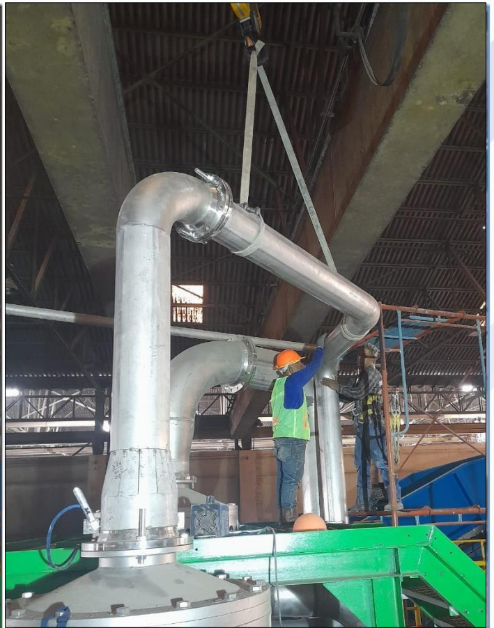
(Piping Instalation stainless steel)
